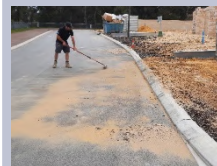
Figure 18: 0.02\text{m}^3 = 30\text{kg} of soil and sand left 446\text{m}^2 lot (R. Davenport, site supervisor, WBN)
