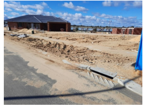
Example of poor site sediment management practices commonly observed during the Perth South West region 'Sediment Snapshot Pilot Trial' (Photo credit: Perth NRM)
