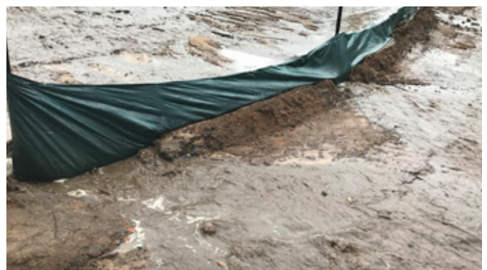
Sediment fences are ineffective if not implemented correctly
